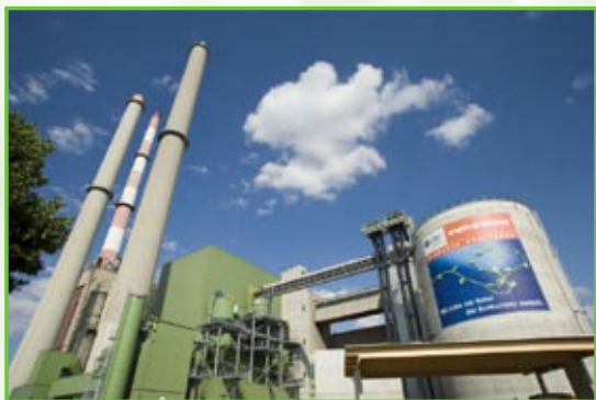
Vienna Biomass Plant
